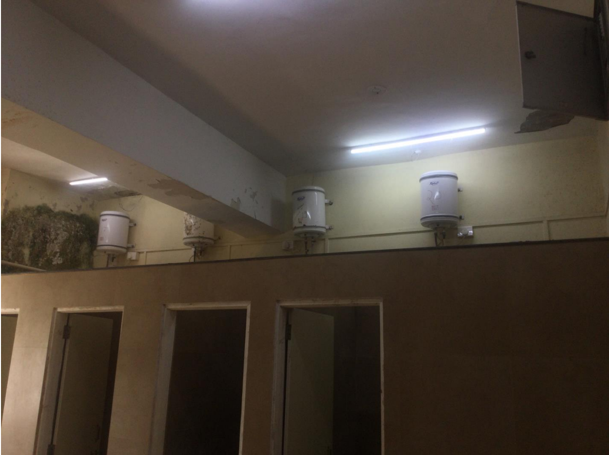
Photo-4: Electric geysers at Bharati Vidyapeeth's College of Engineering, Lavale, Pune
