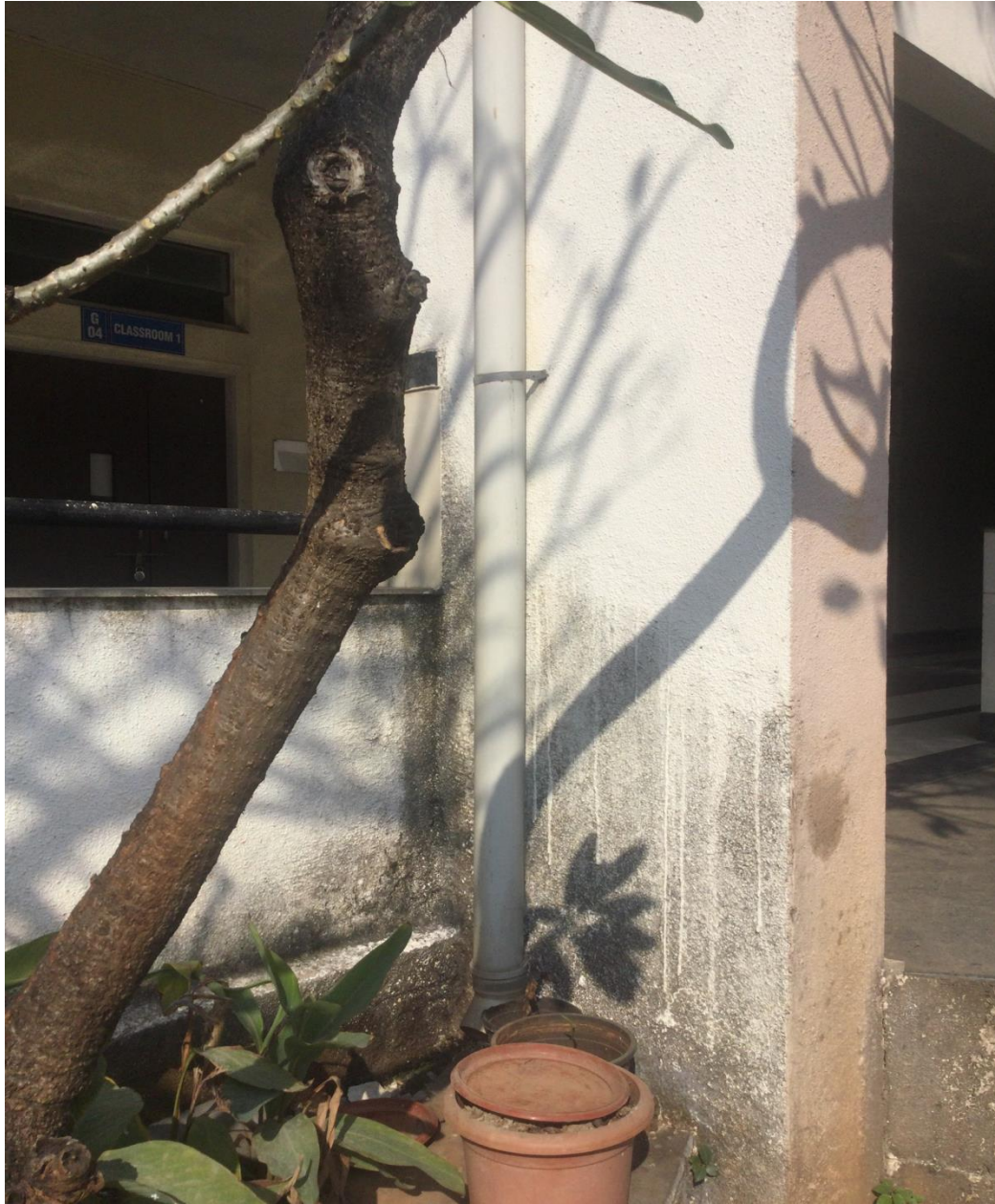
Photo-5: View of rain water collection from building
