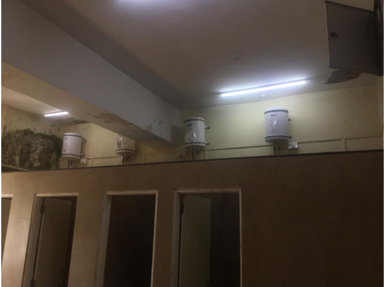
Photo-1: Electric heaters in the boys hotel at BV CoE, Lavale, Pune
