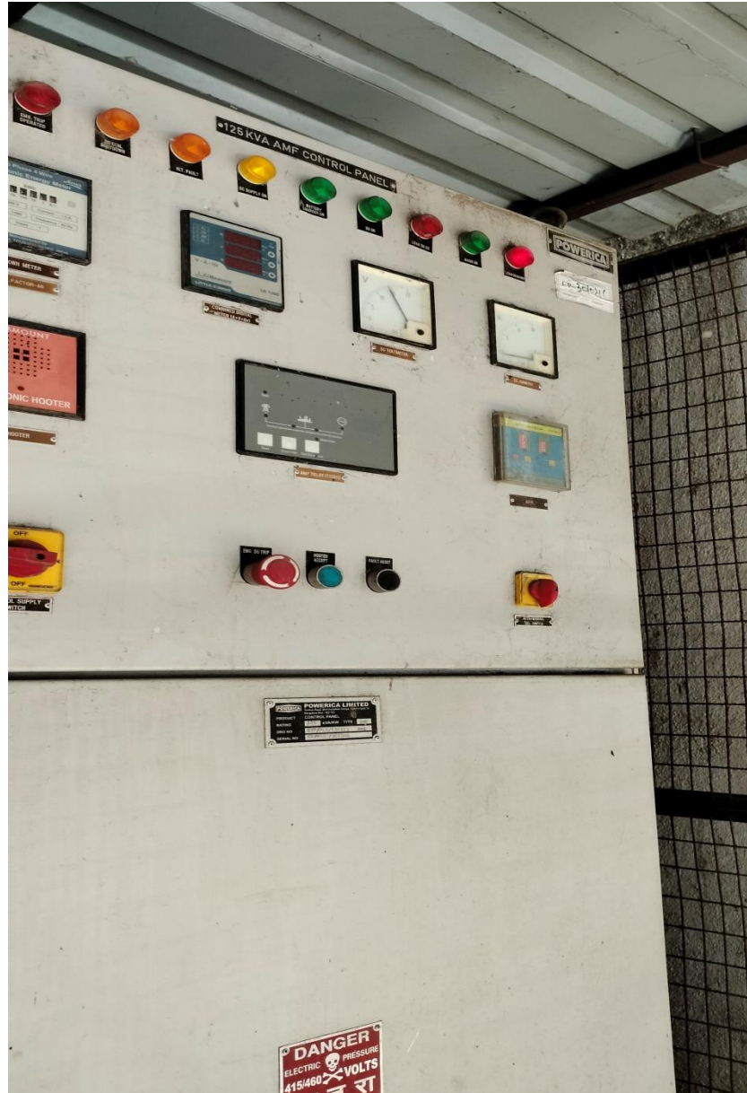
Photo-6: APFC 125kVAR at Bharati Vidyapeeth's College of Engineering campus
