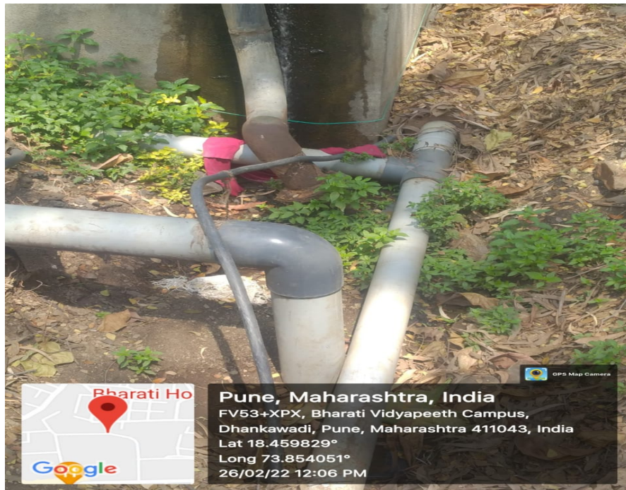
Recycled waste water distribution junction in the campus
